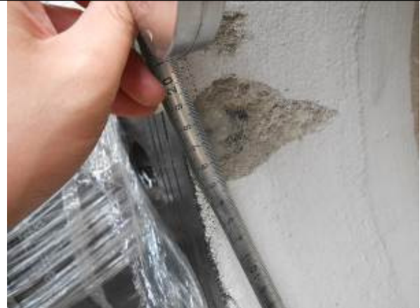
cement fall off
